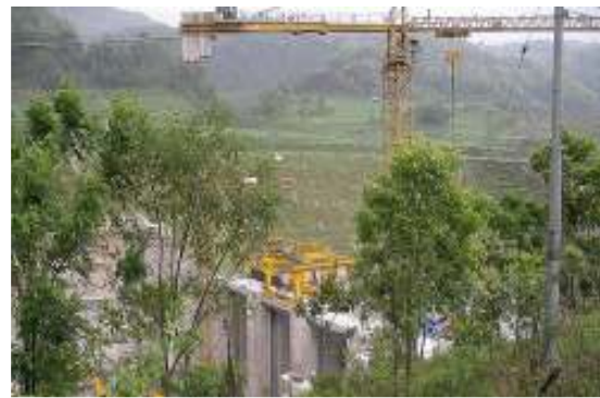
Figure 2: Hydroelectric potential being developed in Nepal
